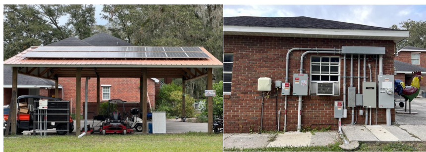
Figure 3 (left) carport solar panel; (right) carport inverter
